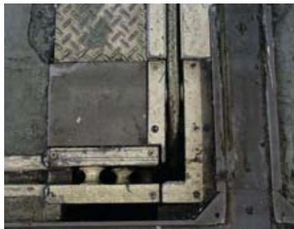
Sharp angle of bolster cable that was used prior to the wireless network
