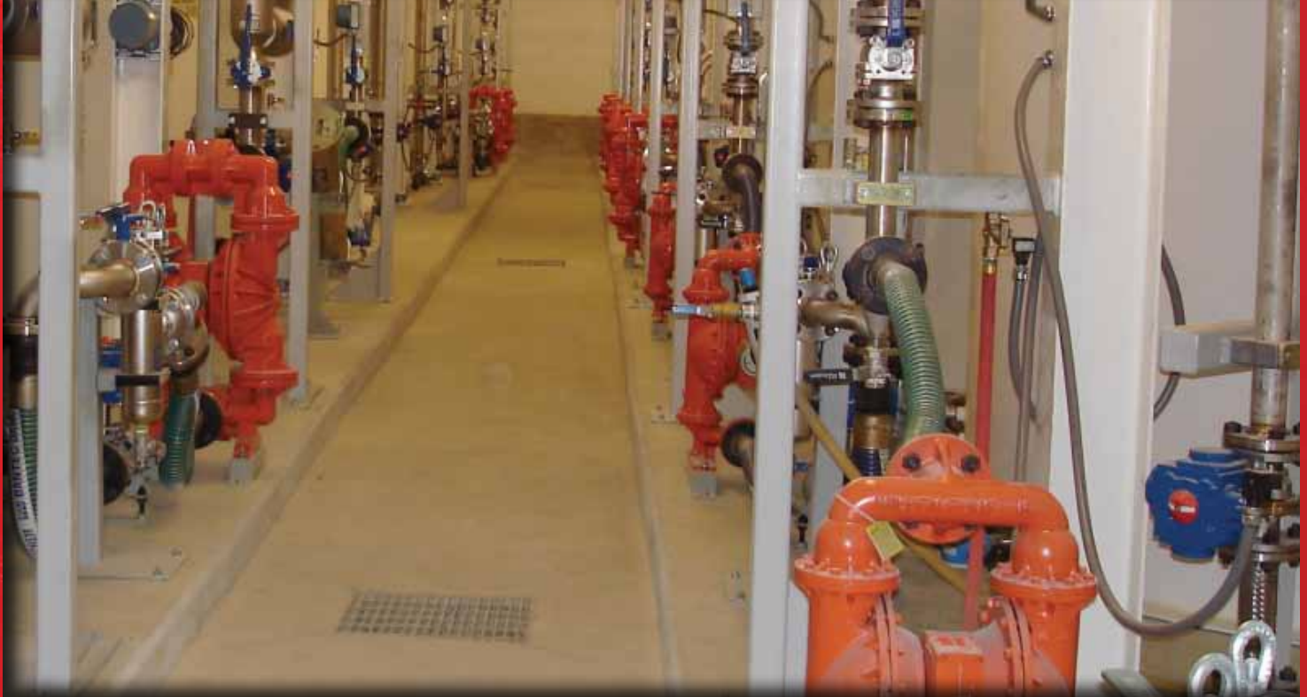
Valspar Tank Farm installation by MMCI. Includes Micro Motion Mass Flow Meters with HART Interface.
