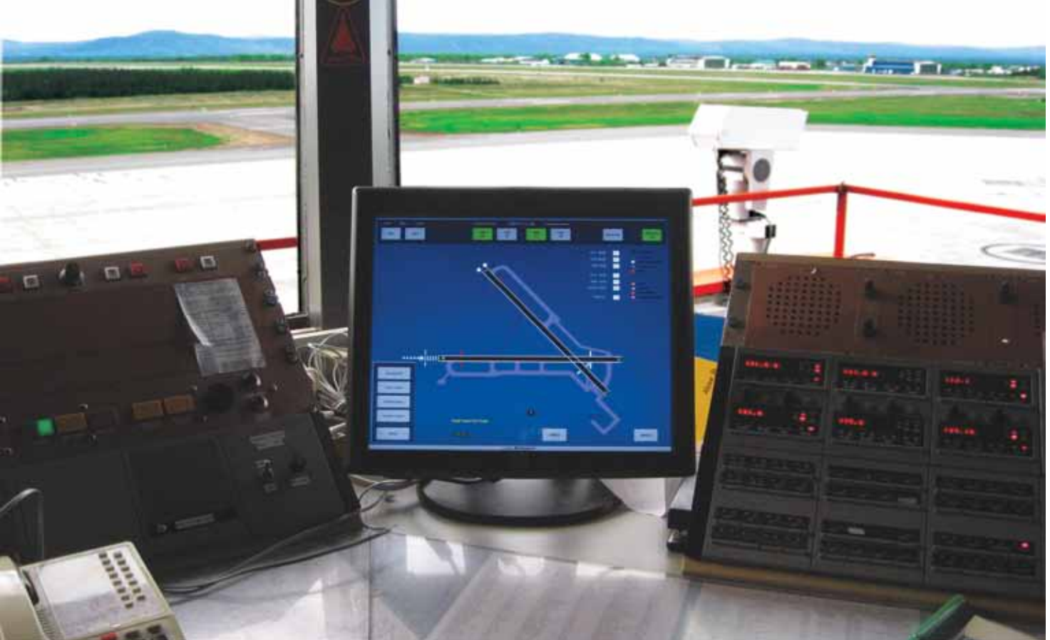
Touch screen Supervisory Control and Data Acquisition (SCADA) operator console located in the Air Traffic Control Tower.
