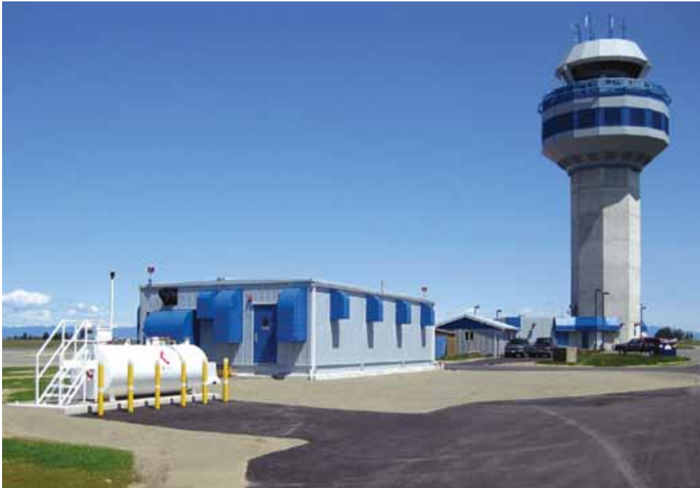
View from the runway of a power vault and Air Traffic Control Tower, which jointly contain the software and equipment that make up the Airfield.
