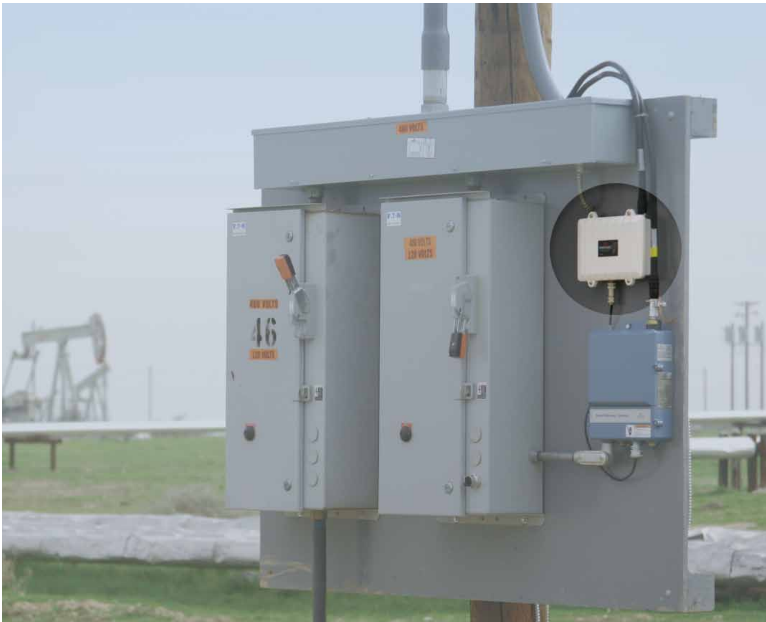
Because of its weather-proof casing, ProSoft's Industrial Hotspot can be mounted outside the panel.
