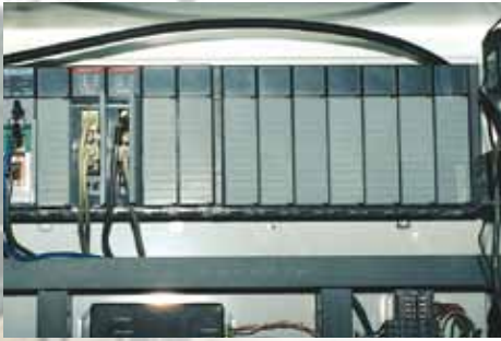
Rockwell Automation processors were installed at each of the five remote well sites containing a ProSoft Technology Modbus Communication Module and a DF1 Communication Module.
