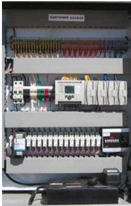
All communication from the wells and injectors to the sub-stations, and from the sub-stations to the Main Master Station, is handled wirelessly using ProSoft Technology's Industrial Hotspot solution.
