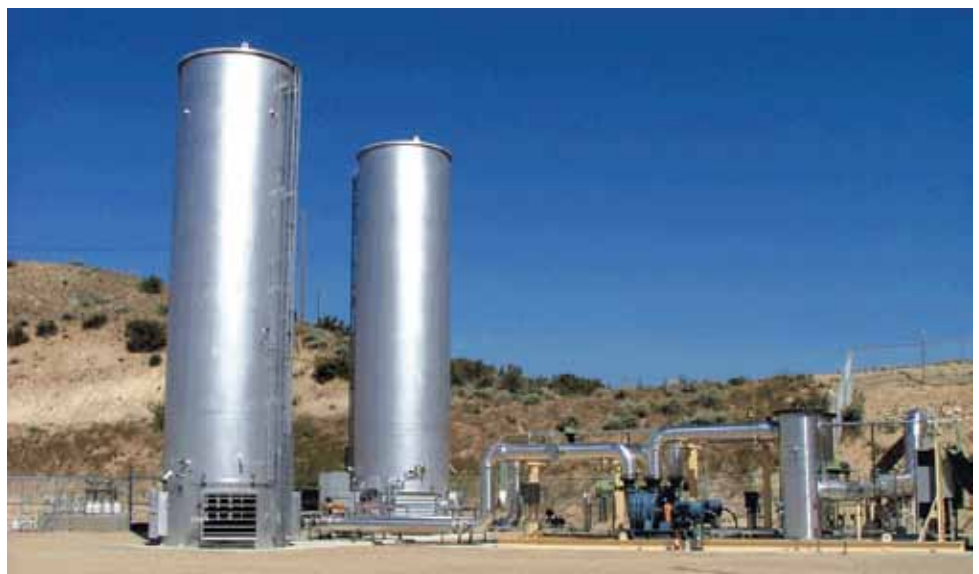
Ada County Landfill's gas extraction system is managed using a ProSoft Technology wireless radio network.
